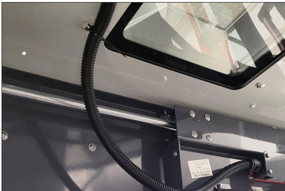
Figure 4-163: Cable routing from the enclosure light to the door, without interference.
