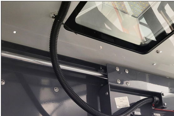
Figure 4-158: Cable routing from the enclosure light to the door, without interference.
