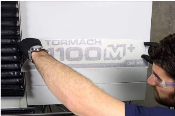
Figure 19: Positioning the new decal on the electrical cabinet.
