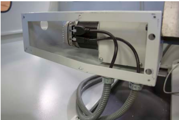
Figure 10: Wire connections on the X-axis motor.
