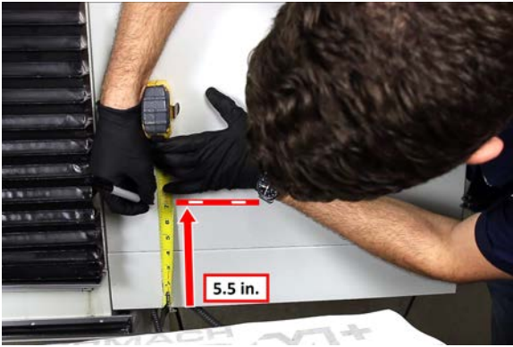
Figure 18: Marking the electrical cabinet for the new decal.
