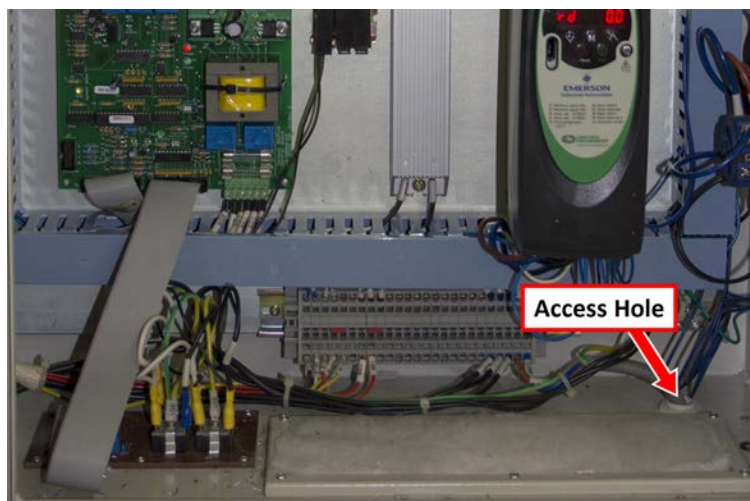
Figure 20: Access hole in the bottom of the electrical cabinet.
