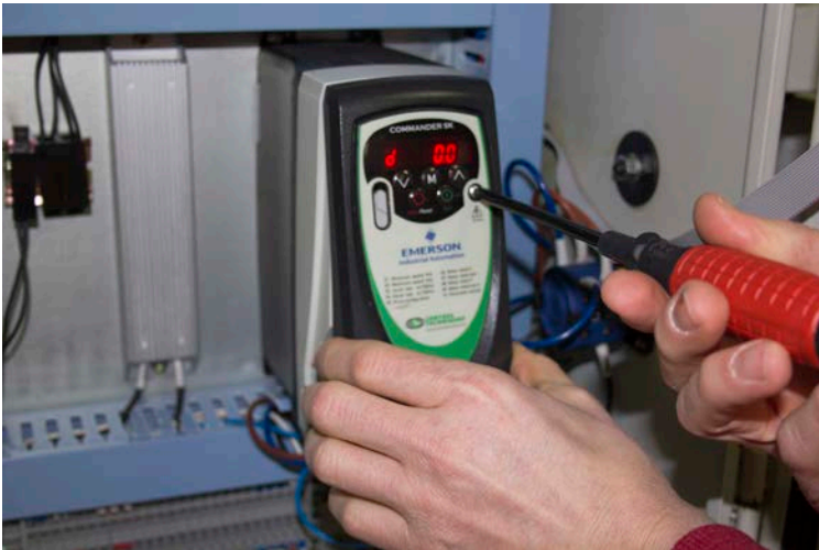
Figure 22: Removing the faceplate from the VFD.
