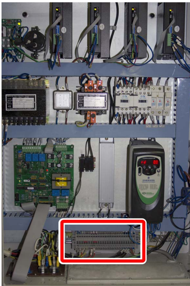
Figure 26: Terminal block in the electrical cabinet.
