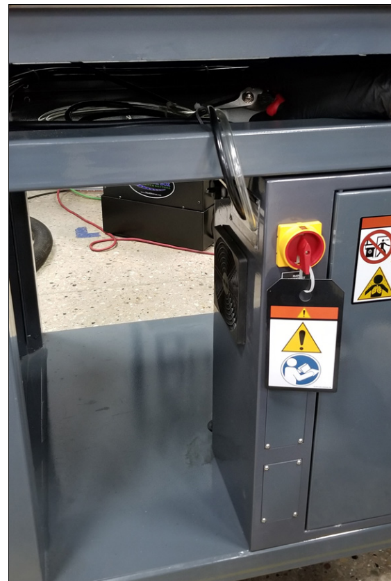
Figure 4-27: The Main Disconnect switch on the side of the machine's electrical cabinet.
