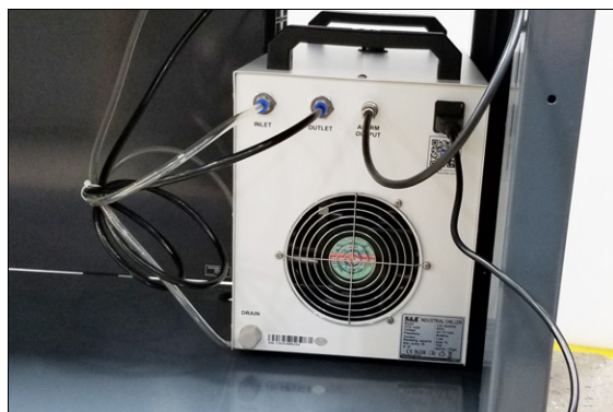
Figure 4-25: Water chiller connections.
