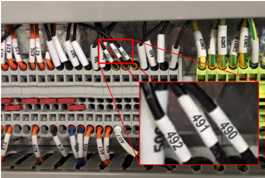
Figure 14: Wires 490, 491, and 492 connected.
