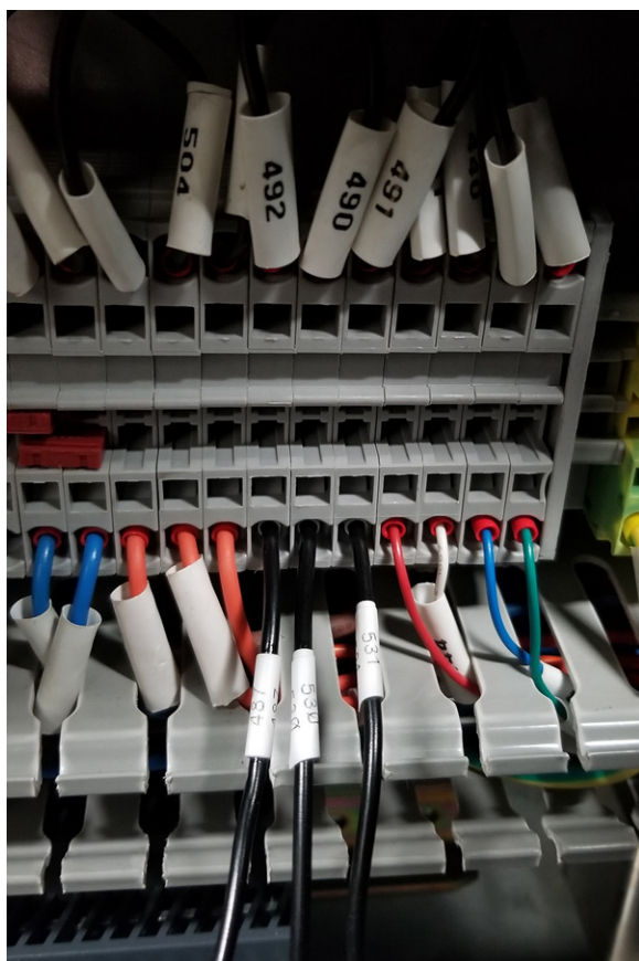
Figure 35: Wires 530 and 531 connected to the terminal block.
