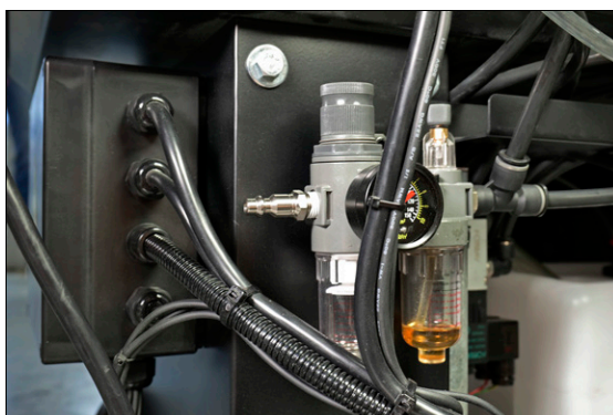
Figure 4-18: Provided air fitting installed on the FRL.
