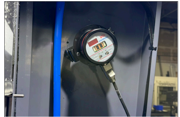
Figure 4-266: Cable connected to the wireless receiver.
