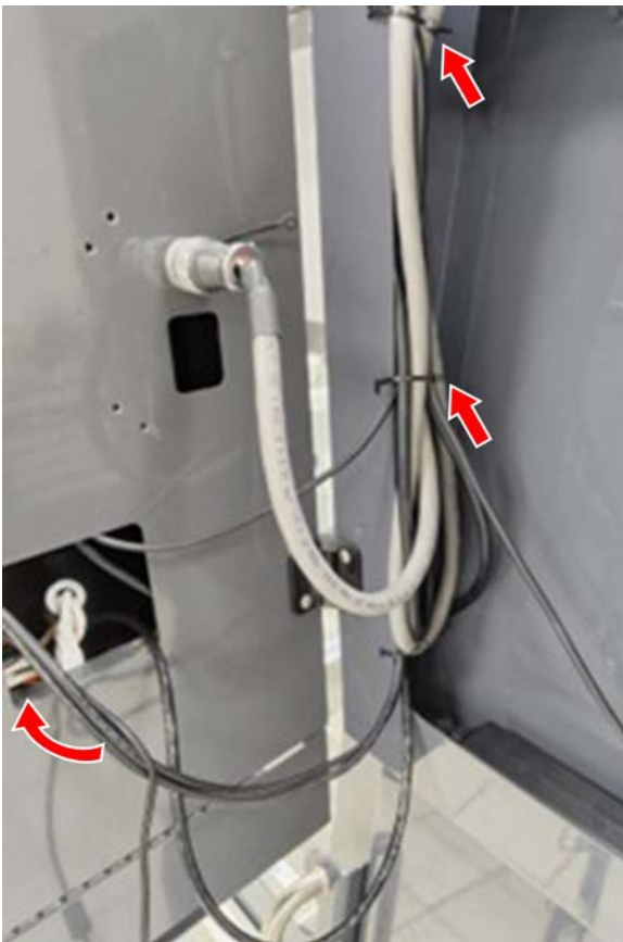
Figure 6: Example of the final cable routing.
