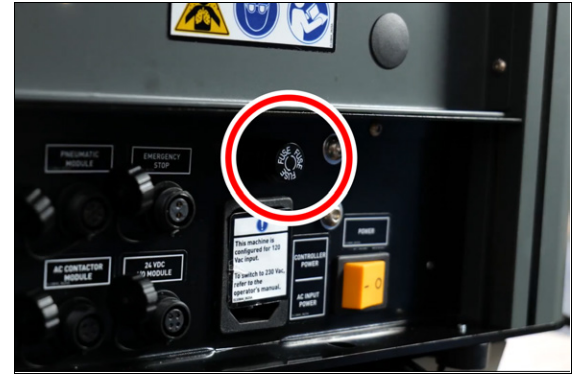
Figure 3-14: Fuse holder on the back panel of the machine.
