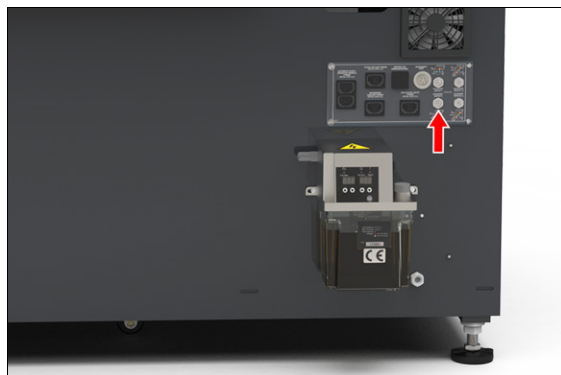
Figure 5-59: Electrical connections panel on the back of the machine stand.
