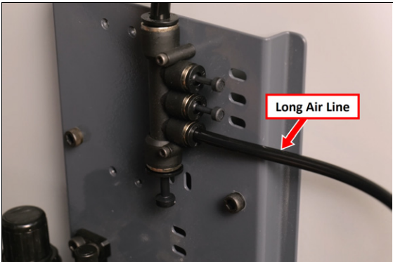
Figure 5-25: Air line connected to the pressure regulator panel.
