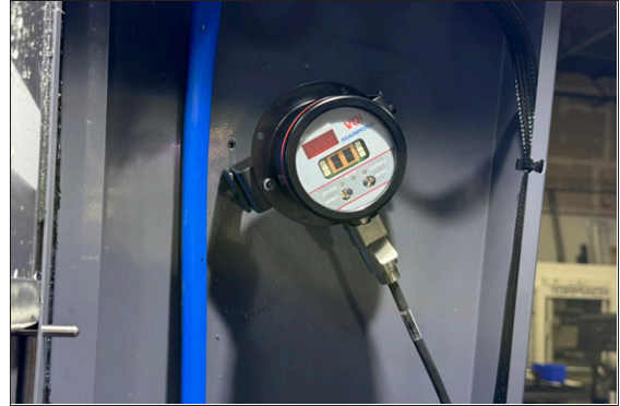
Figure 4-115: Cable connected to the wireless receiver.
